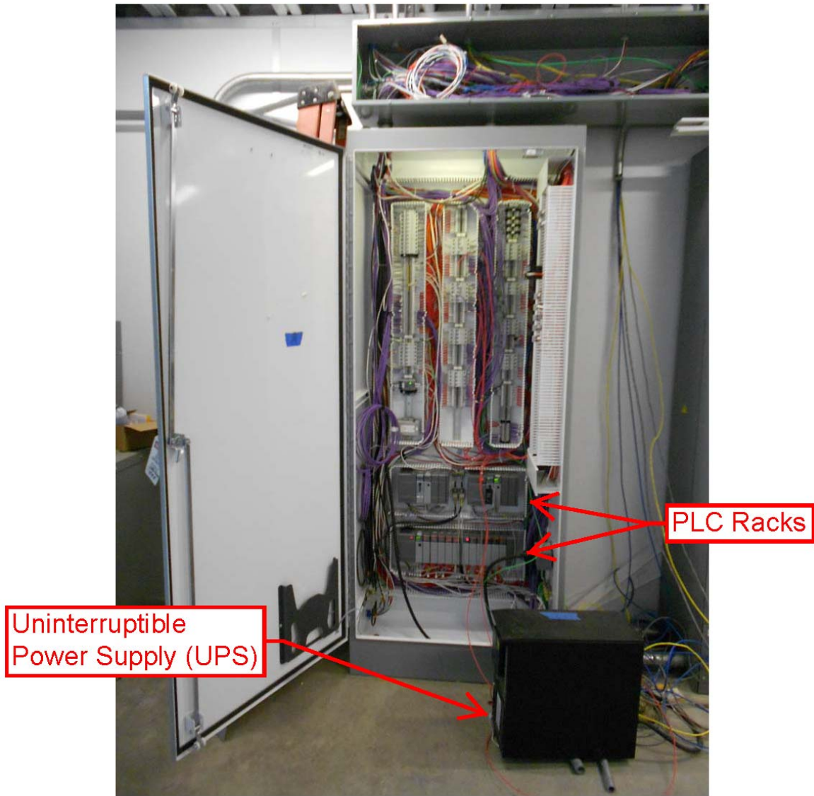
CONTROL PANEL CP-2
